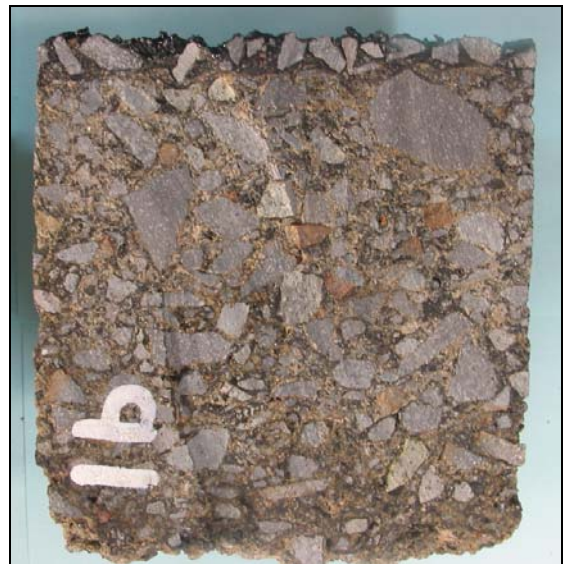
Figure 7: A 150 mm diameter foamed bitumen treated basecourse core cut in half. The stones at the top represent the chipseal
